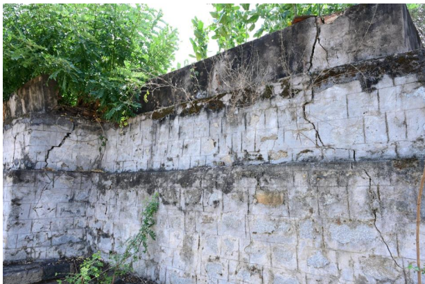
Cracks and separation in later walling
