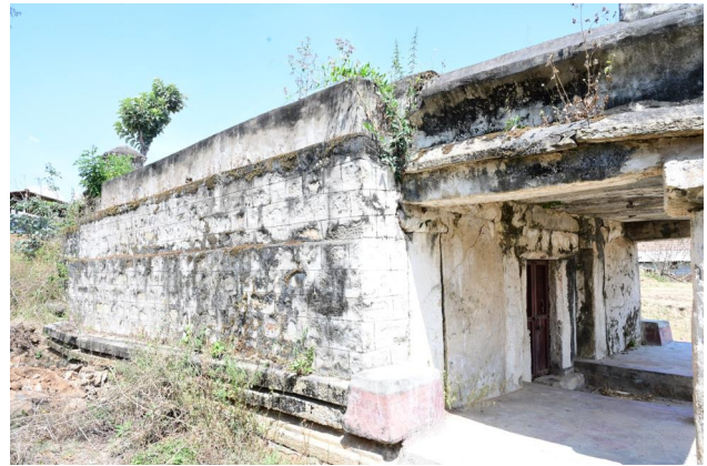
Side elevation showing masonry additions and deterioration.
